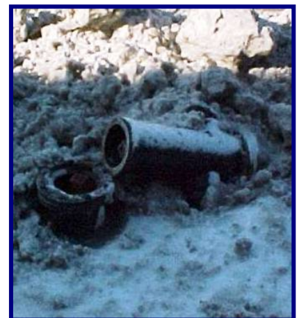
Broken or buried hydrants pose a significant public safety risk.
