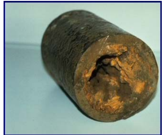
Severely tuberculated pipe can harbor bacteria and put public health at risk.
